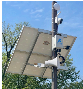
P2P W/ LTE FAILOVER
