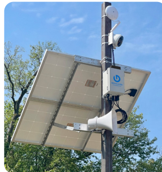
P2P W/ LTE Failover
